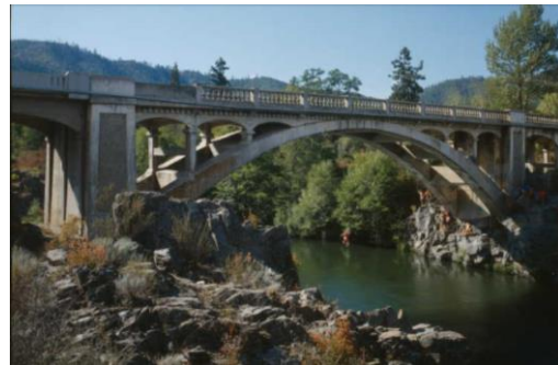
Rock Point Arch Bridge, Spanning Rogue River & Old Pacific Highway, Route 271, Gold Hill, Jackson County, Oregon, 1968 [From the Library of Congress Photo Collection, 1840-2000 on Ancestry ]
